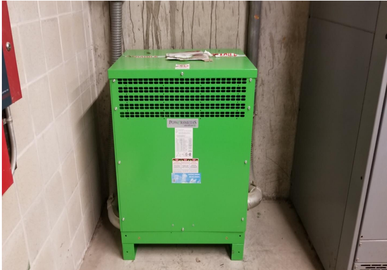
Transformer at the Murray Center
